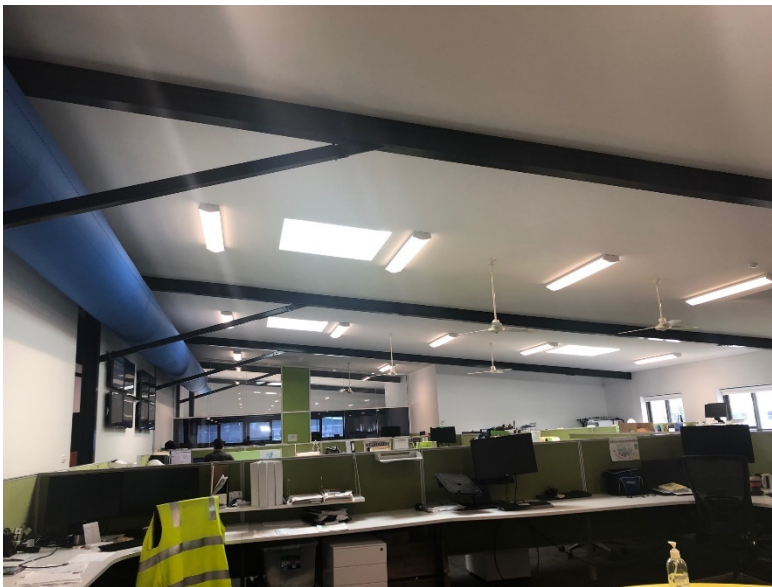
Figure 3 Hobart Airport Administration LED lighting
