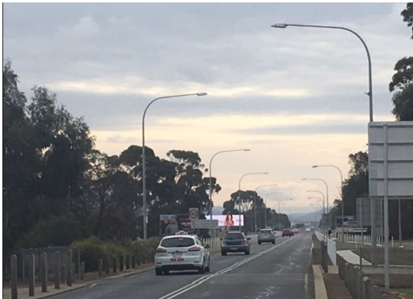
Figure 2 Holyman Ave LED Lighting
